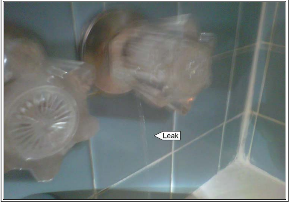
Leak at 2nd floor hall bathroom tub (faucet stem).
