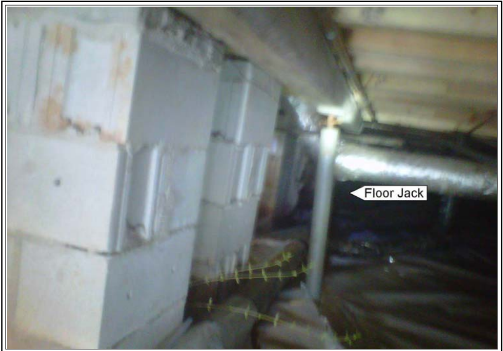
Left side sill has been replaced in crawl. Floor jacks installed for extra support.
