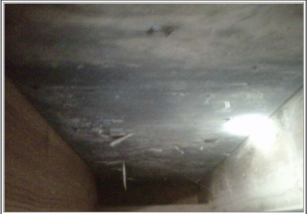
Black stains on sheathing located attic. Possible smoke stains.
