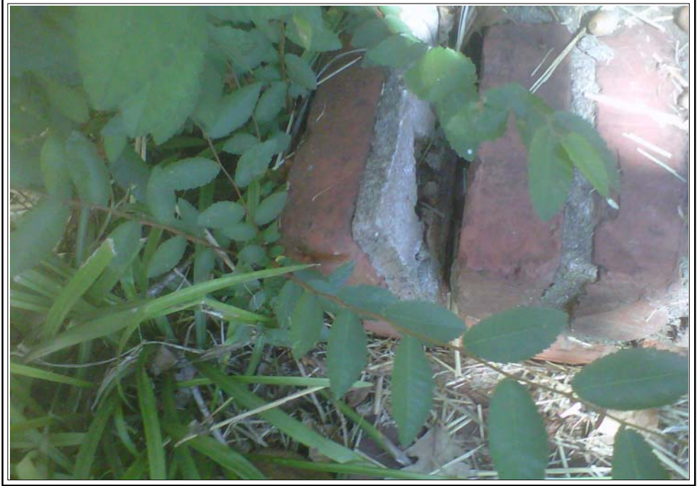
Loose and missing bricks at stoop.
