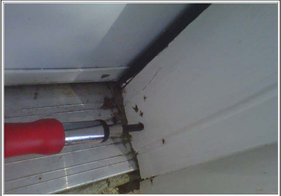
Wood rot at left door casing.
