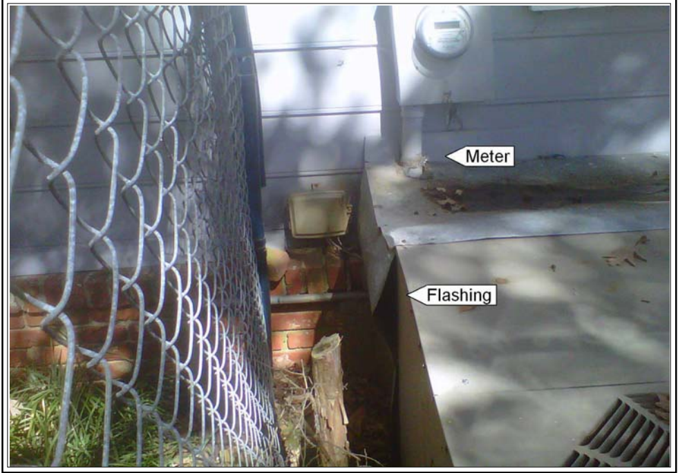
Damage flashing at HVAC unit.
