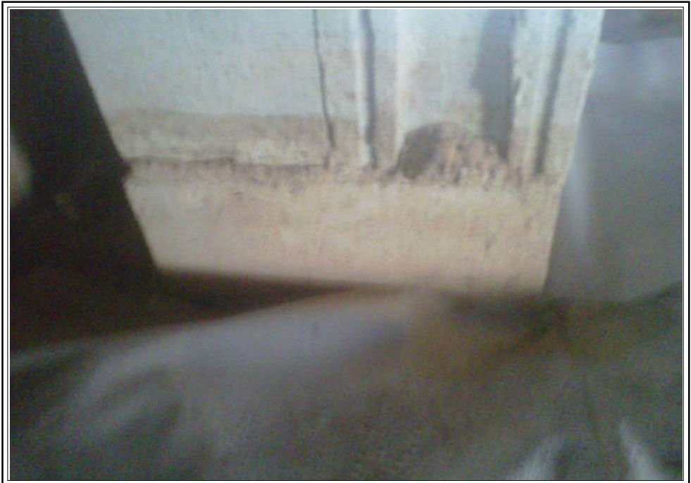
Evidence of past moisture invasion at crawl space.
