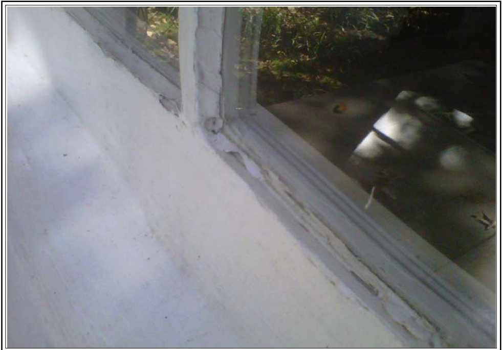
Missing and cracking glazing at breakfast window.
