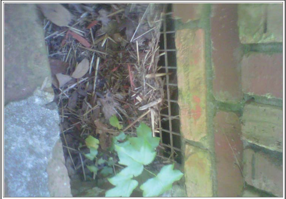
Evidence of moisture invasion at left rear foundation vent.
