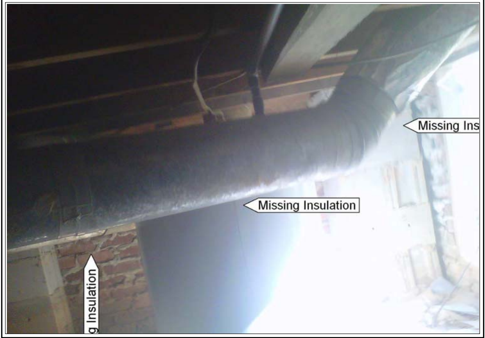
Missing insulation on metal duct work.
