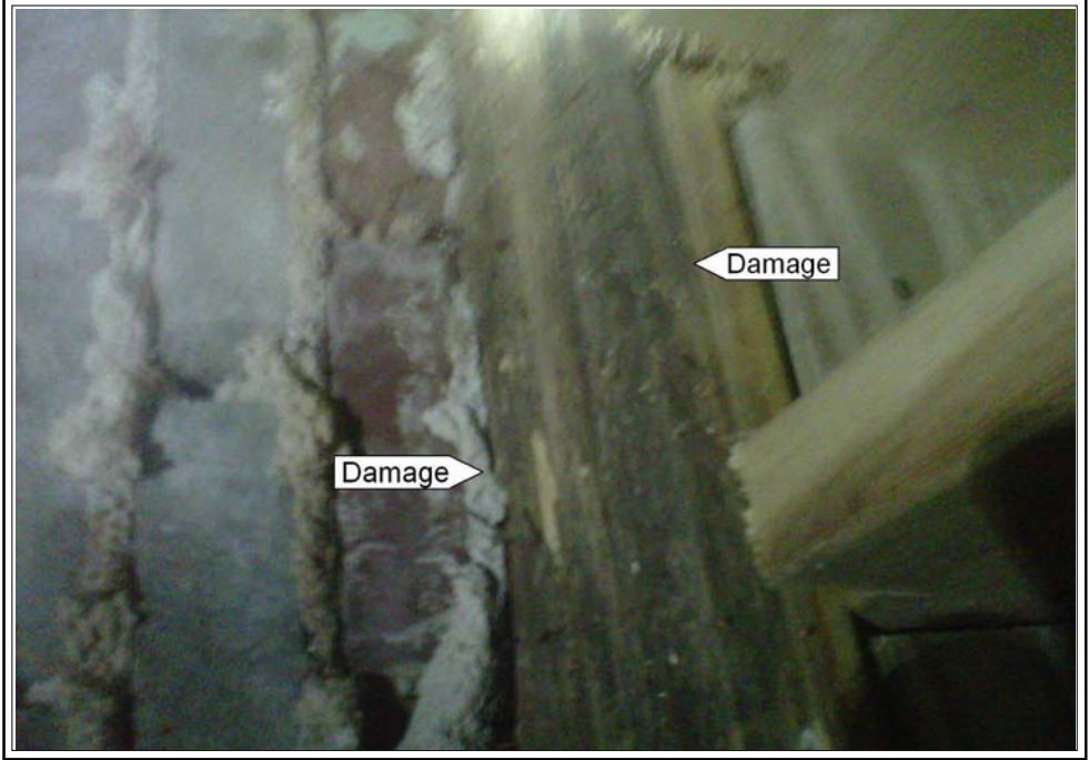
Evidence of damage sill located at front stoop area (crawl space).
